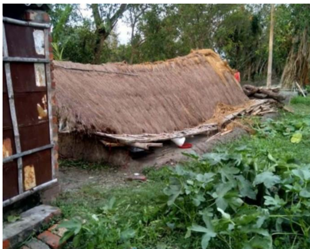
Thatched roof collapsed onto home
